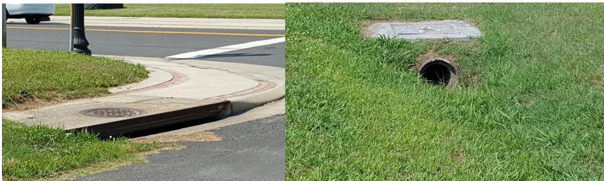
Storm sewer features in downtown Exmore. A-NPDC staff photo.
